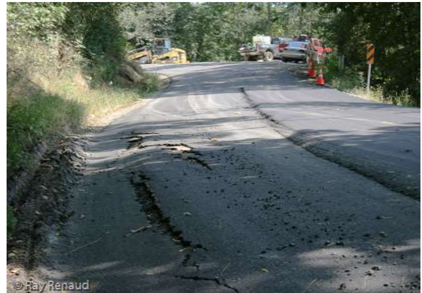
Above : Road Disintegration from Truck Traffic
